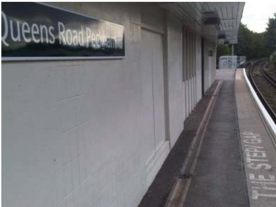
(14) Platform level alongside central block, on northbound platform, showing narrow platform width and sight lines obscured including entrance/exit, 16/9/09
