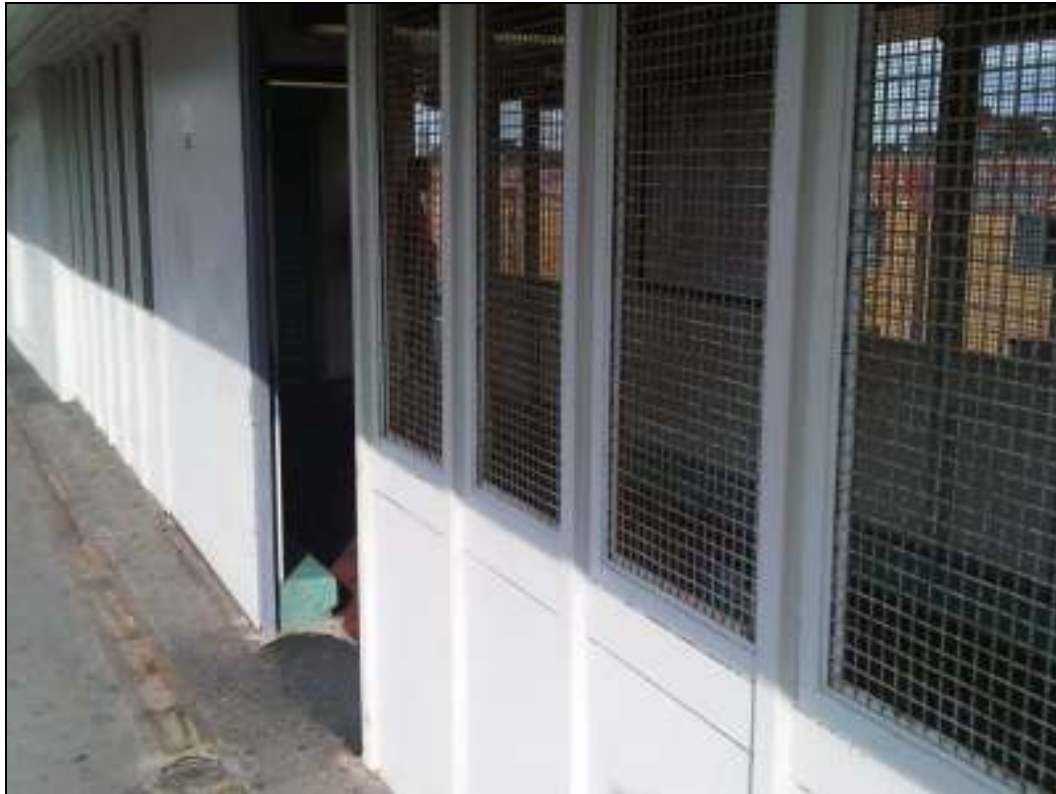
(13) Booking office and circulating area at top of staircase, and open grilles in window frames, seen from northbound platform, 16/9/09
